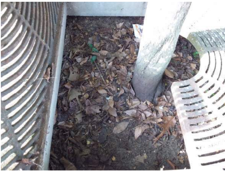
BMP #13- inside filterra
