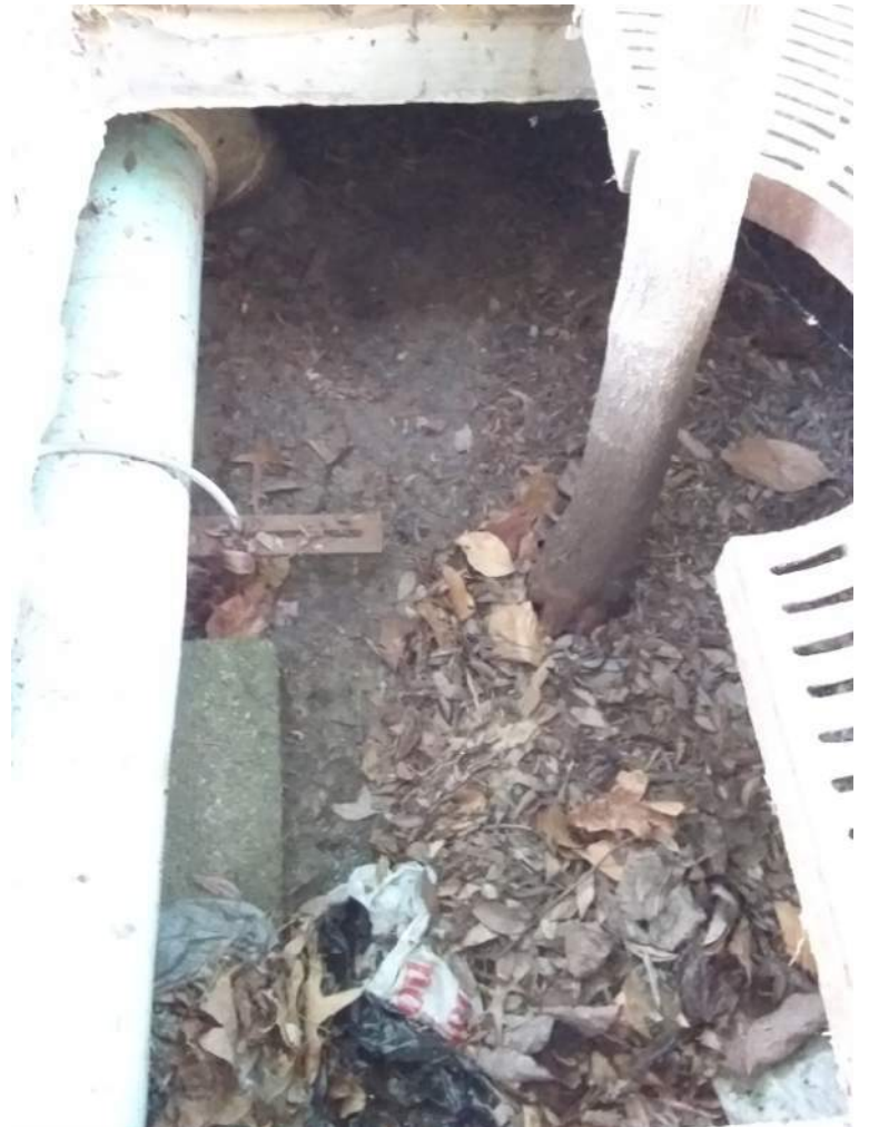
BMP #2- inside filterra
