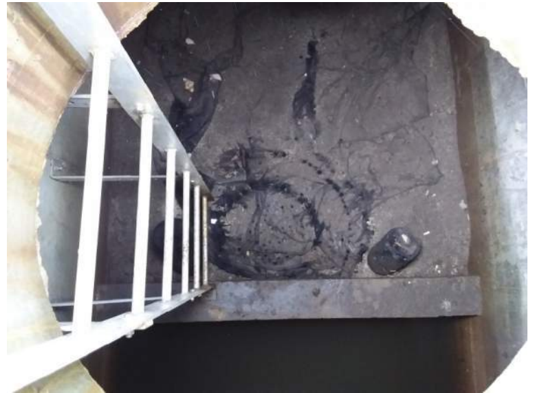
BMP #27- inside view of sand filter side
