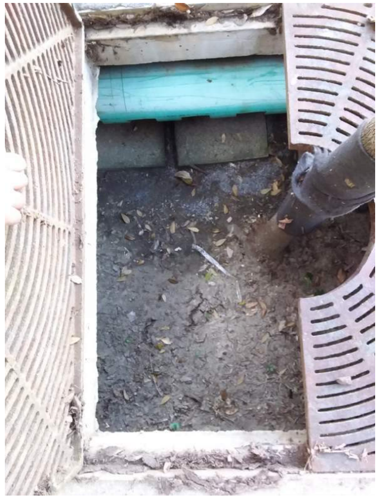
BMP #3- inside filterra
