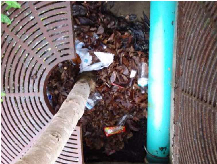
BMP #20- inside filterra
