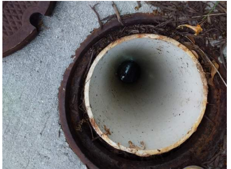
BMP #36- inside view
