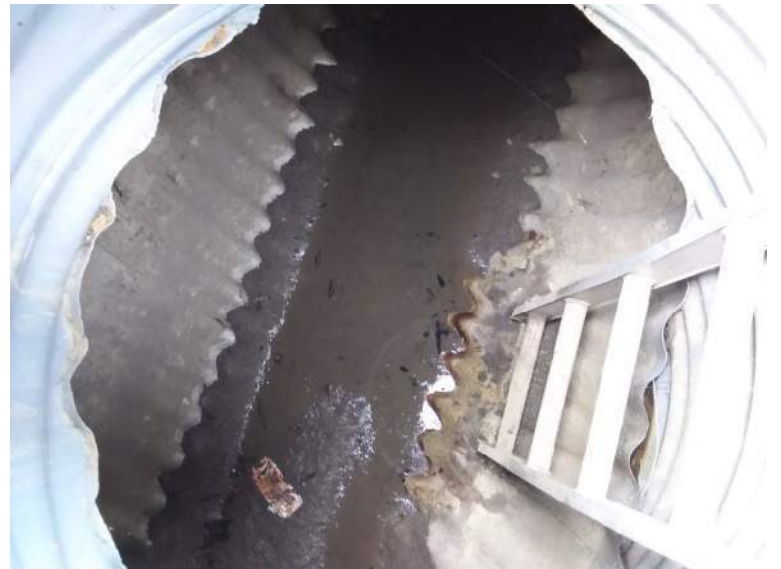
BMP #25- inside view
