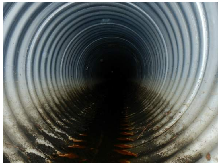
BMP #40- inside view
