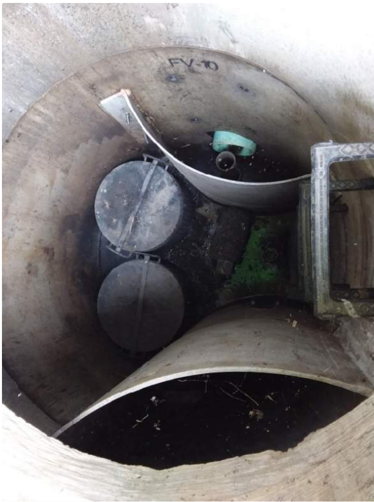
BMP #34- inside view
