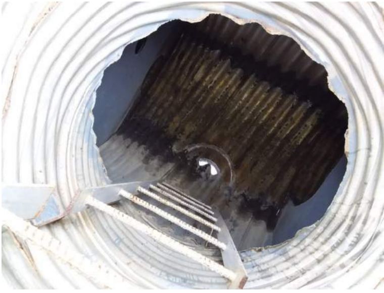
BMP #50- inside view
