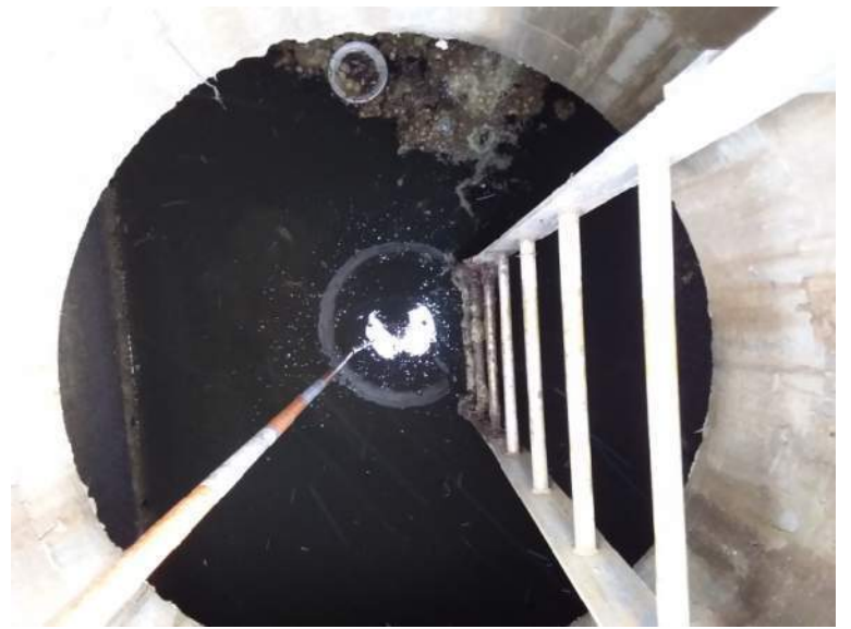
BMP #28- inside view of detention chamber
