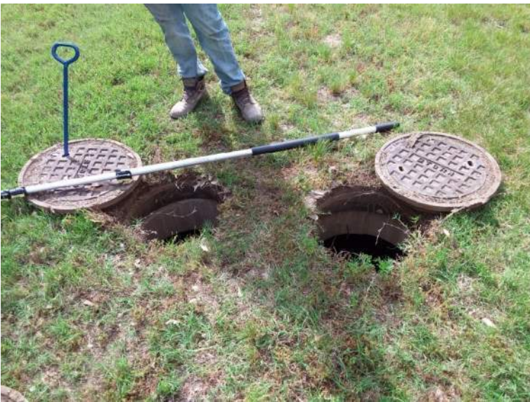
BMP #31- right manhole is access to the sediment chamber, left manhole is access to the sand filter side
