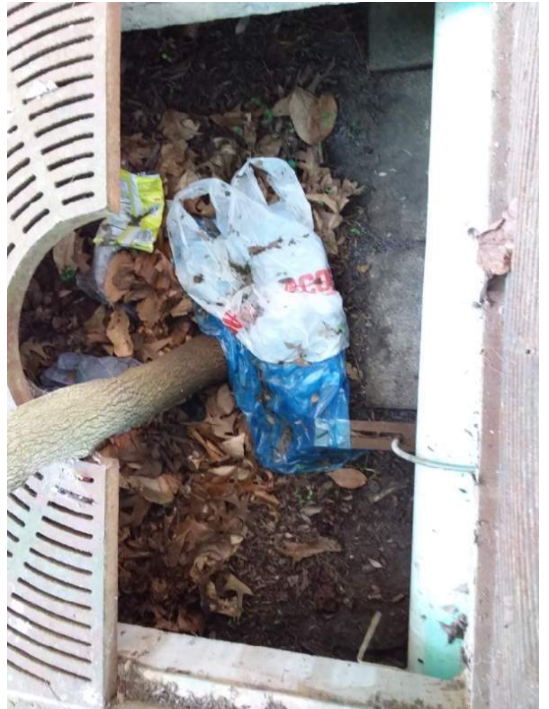
BMP #4- inside filterra
