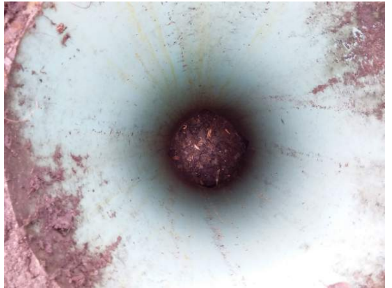
BMP #38- inside view
