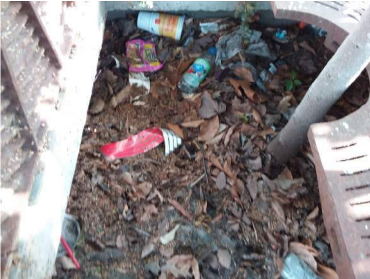
BMP #7- inside filterra
