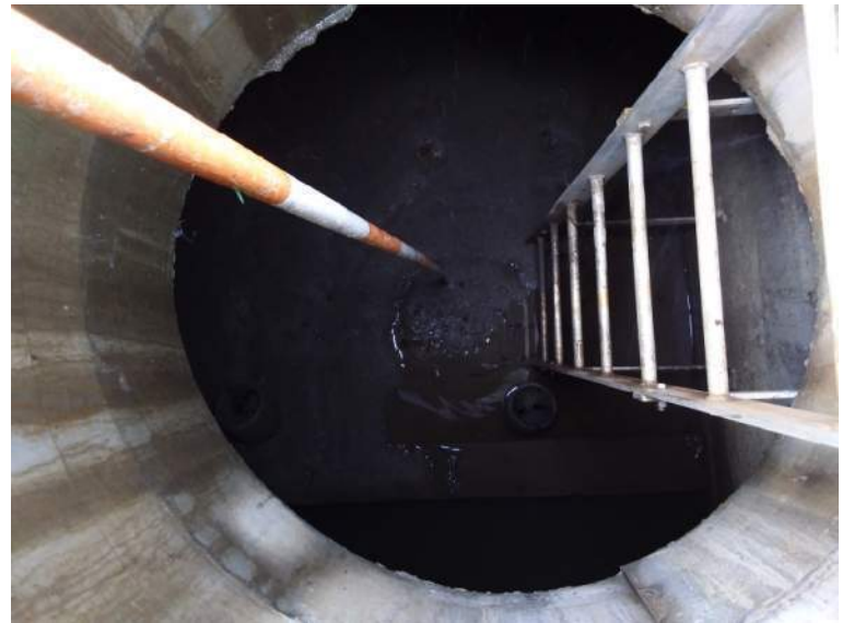
BMP #28- inside view of sand filter side
