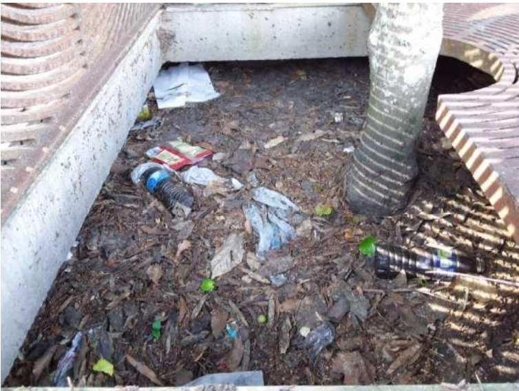
BMP #9- inside filterra
