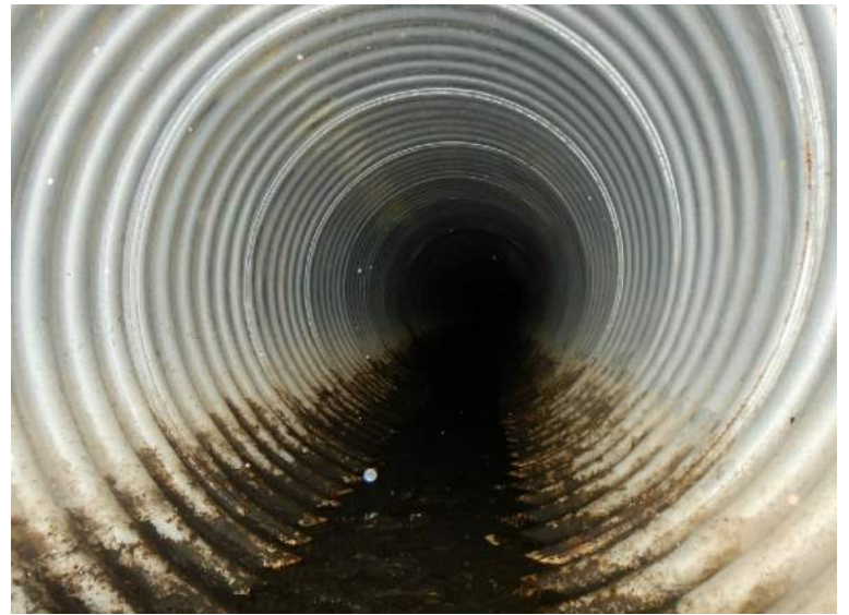
BMP #15- inside view
