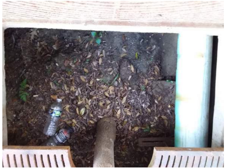
BMP #5- inside filterra
