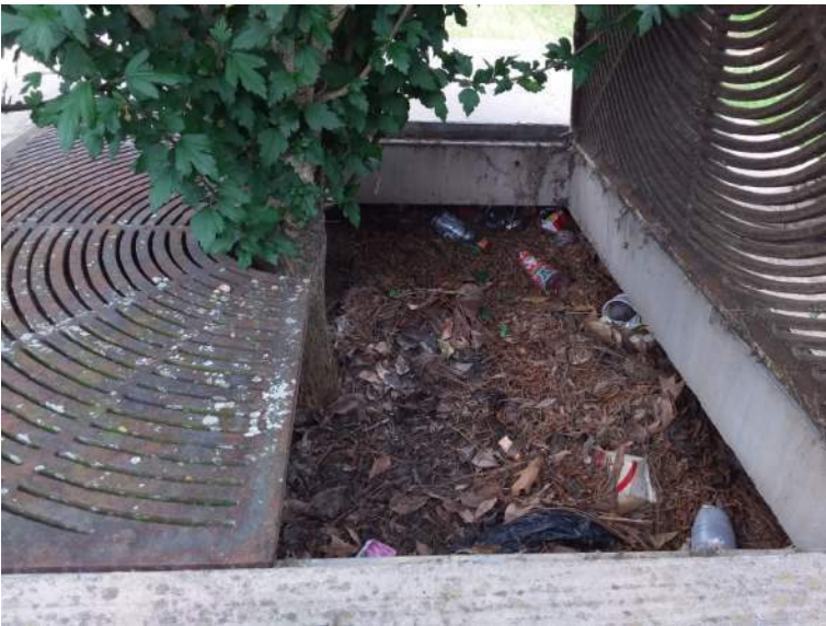
BMP #43- inside filterra
