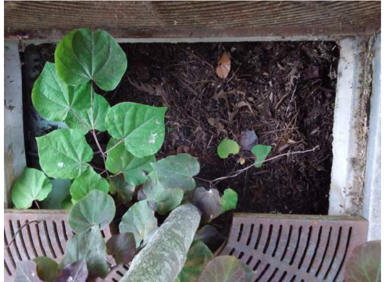
BMP #6- inside filterra
