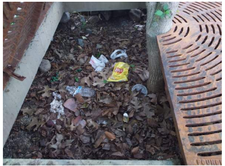
BMP #42- inside filterra
