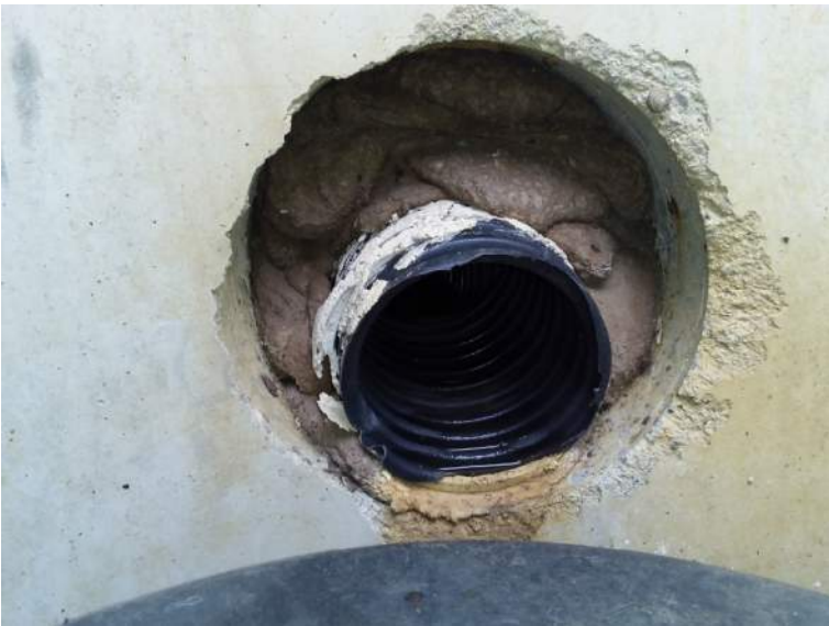
BMP #35- inlet pipe needs to be mortared
