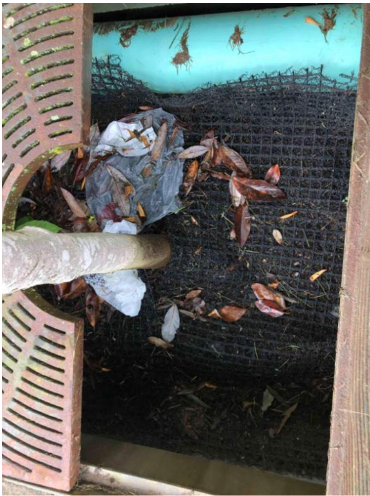
BMP #16- inside filterra
