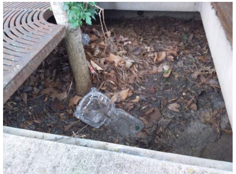
BMP #41- left side of filterra
