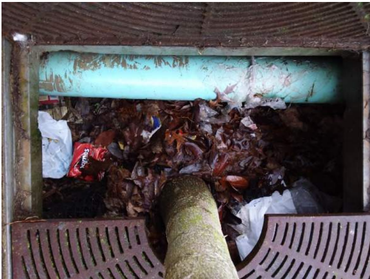
BMP #18- inside filterra
