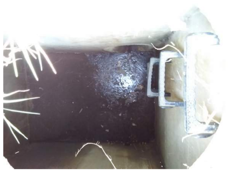
BMP #31- inlet chamber
