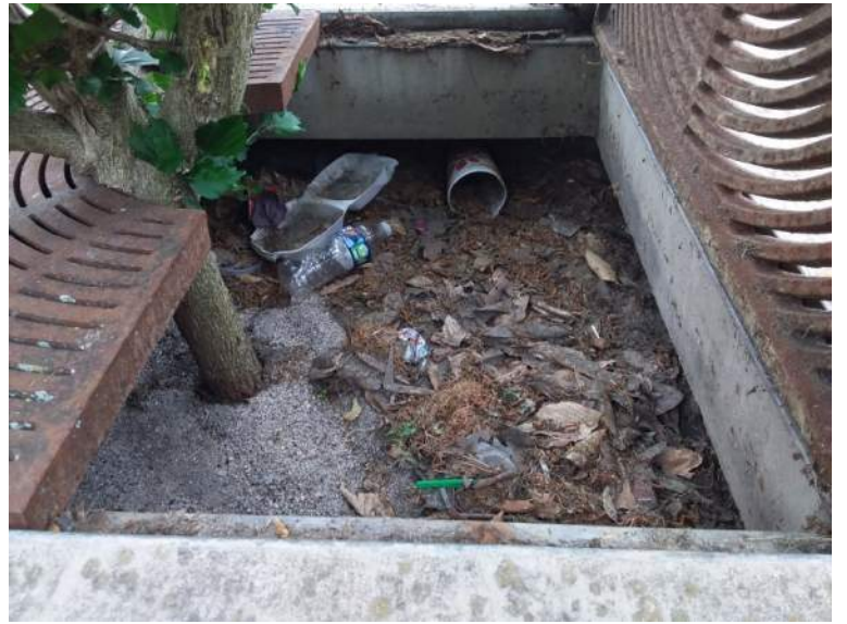
BMP #44- inside filterra
