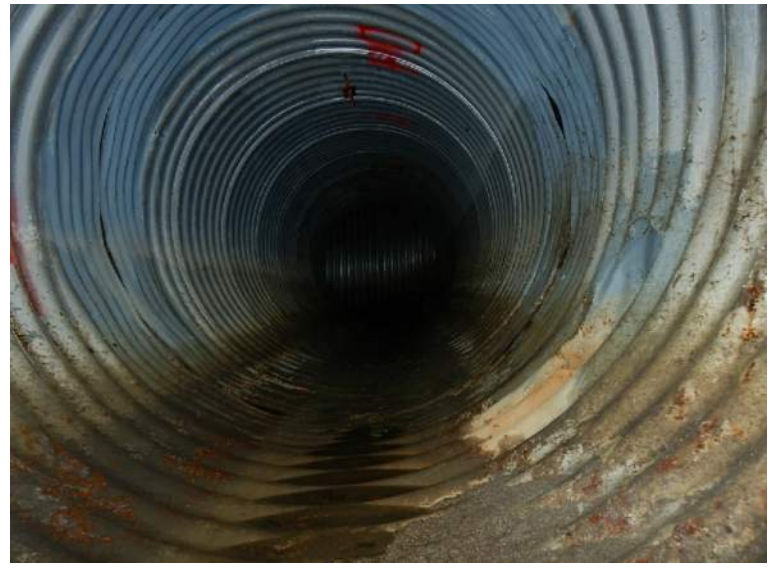
BMP #26- inside view
