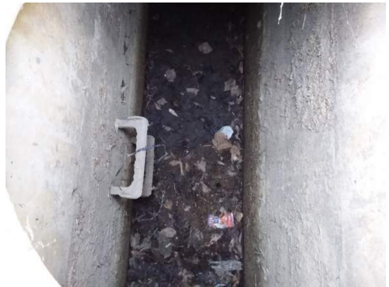
BMP #31- sediment chamber
