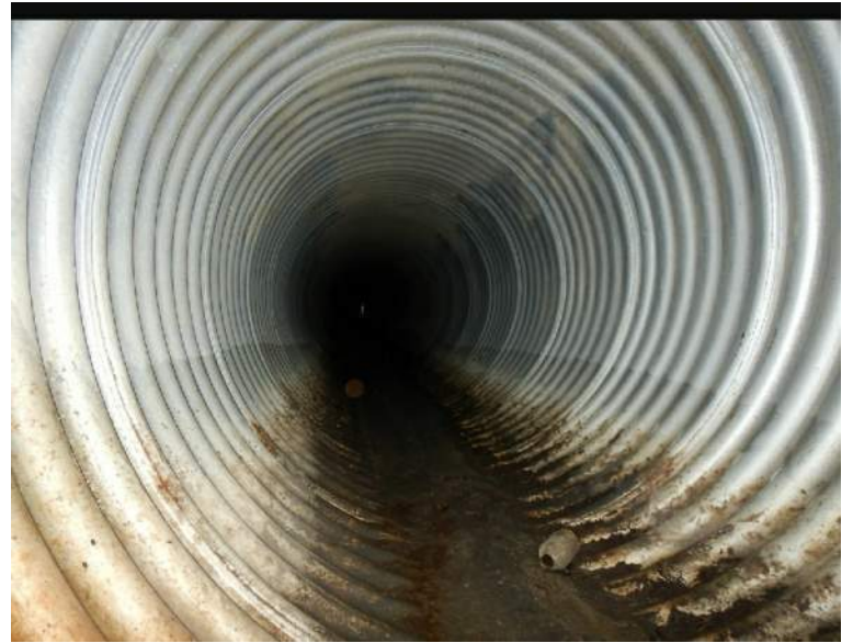
BMP #15- inside view
