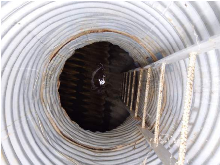
BMP #50- inside view
