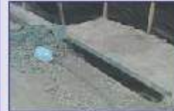
Failed Inlet Protection
