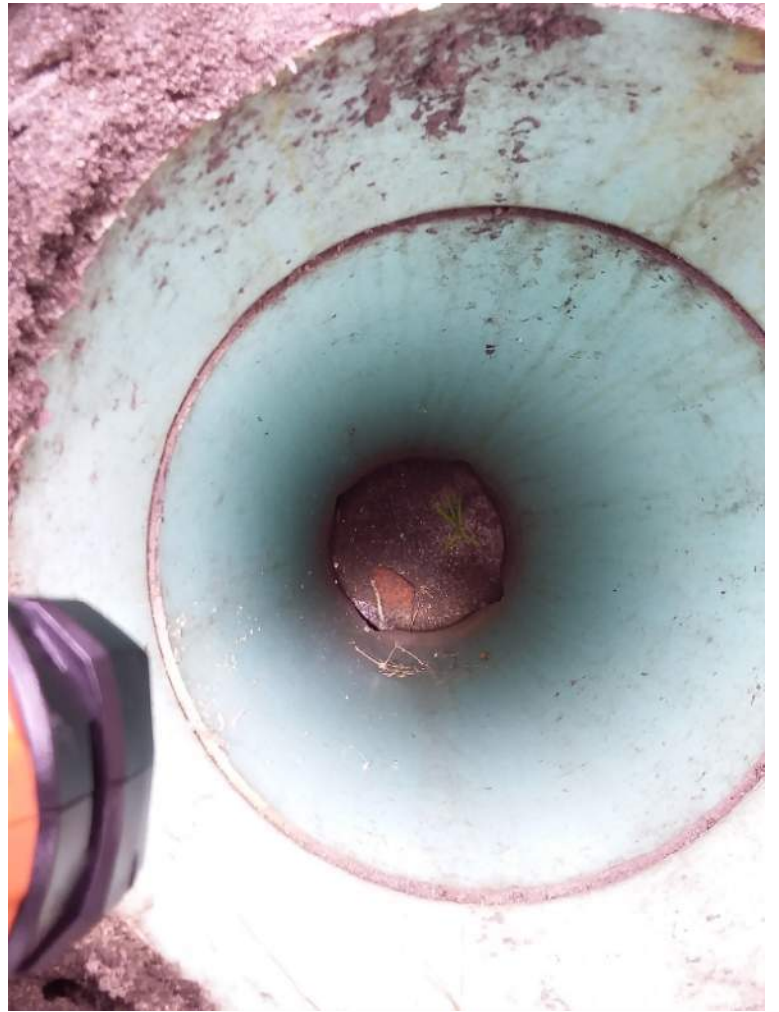
BMP #37- inside view
