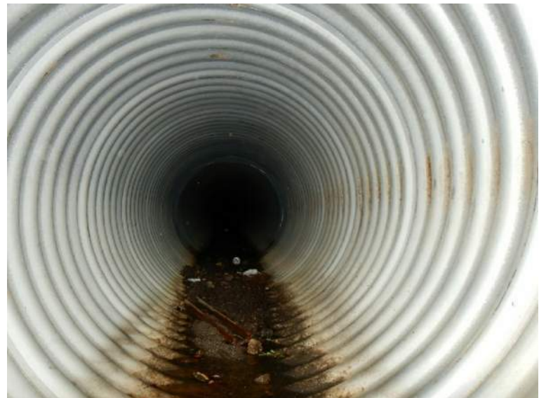
BMP #15- inside view
