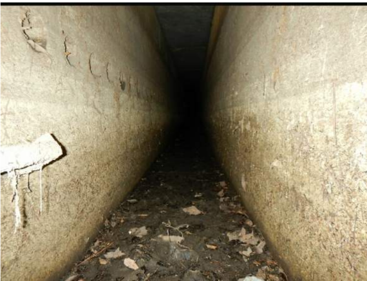
BMP #31- sediment chamber
