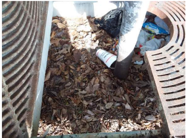
BMP #12- inside filterra
