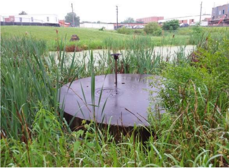
BMP #30- outlet structure
