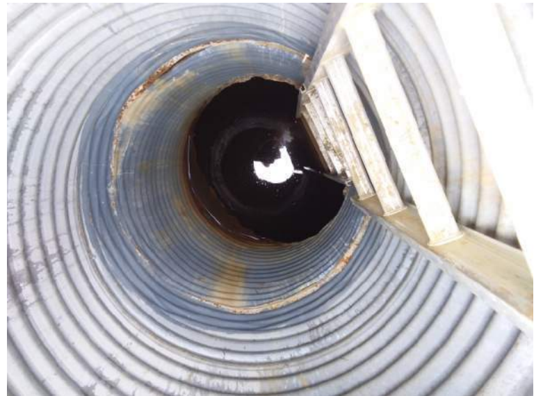
BMP #24- inside view
