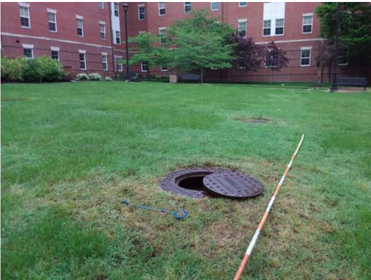
BMP #27- top view of detention chamber
