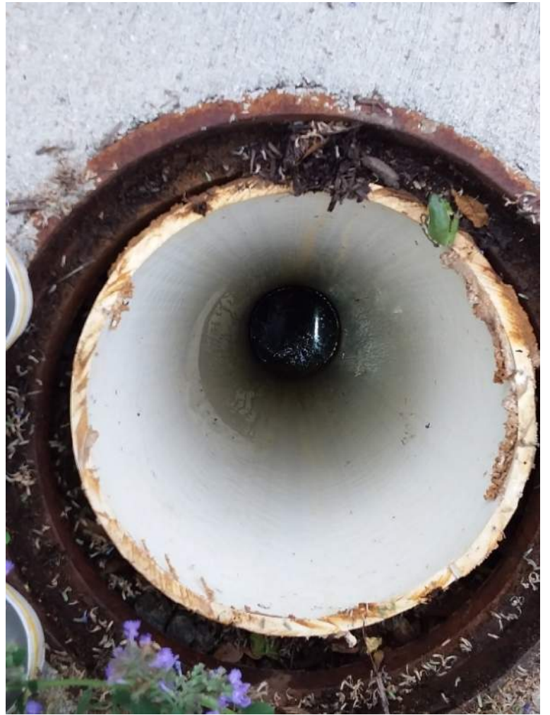
BMP #36- inside view
