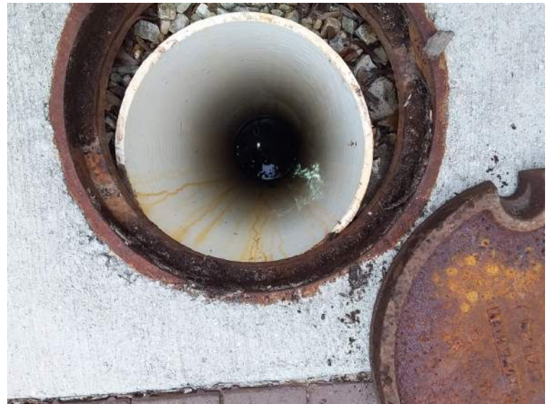
BMP #36- inside view
