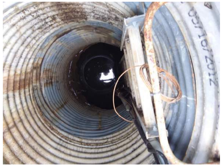
BMP #24- inside view
