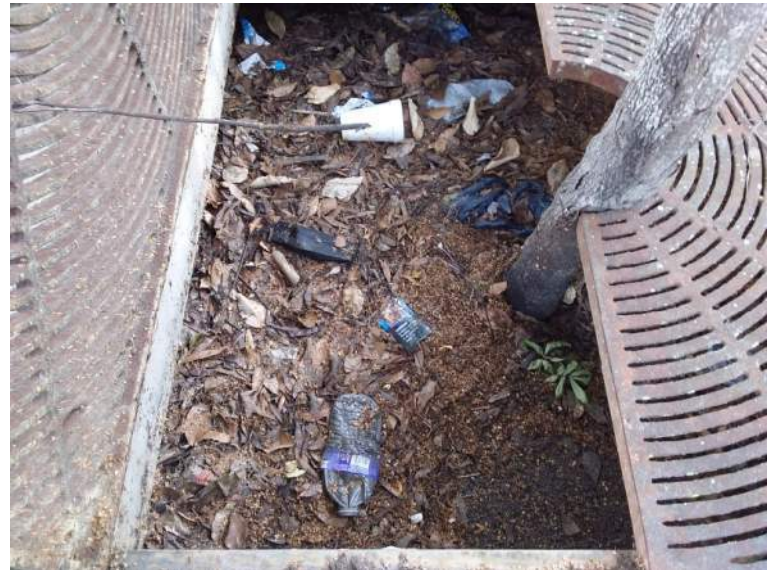
BMP #8- inside filterra
