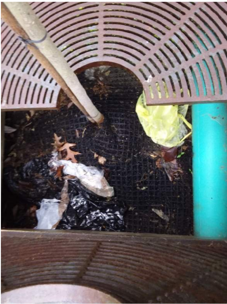
BMP #19- inside filterra
