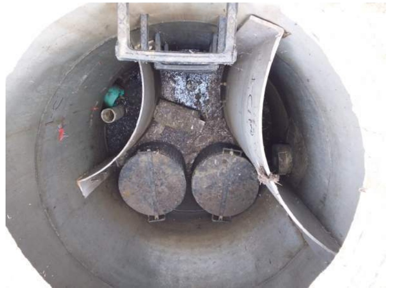
BMP #33- inside view
