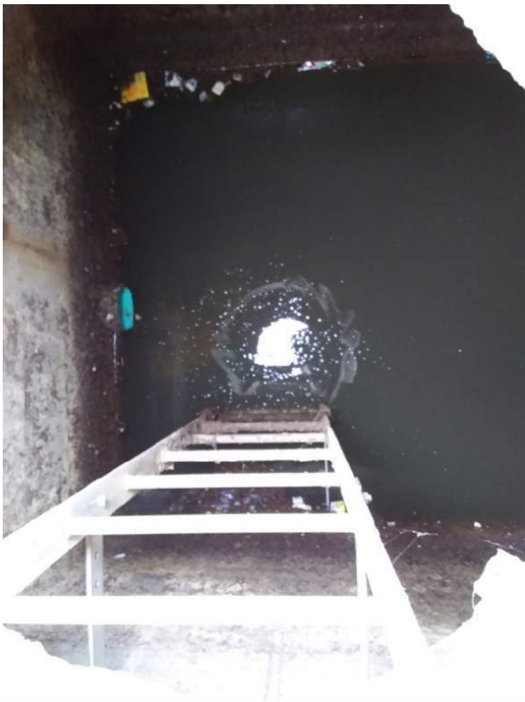
BMP #27- inside view of detention chamber
