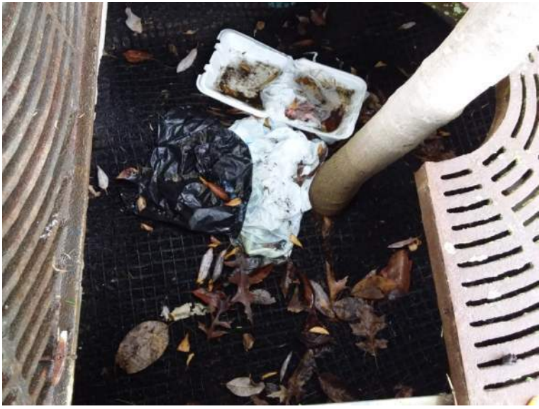
BMP #21- inside filterra
