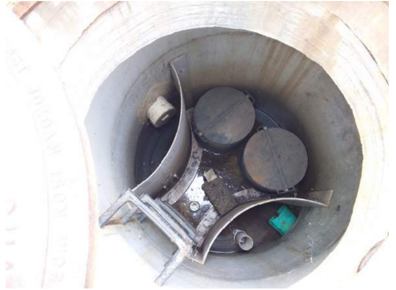
BMP #32- inside view
