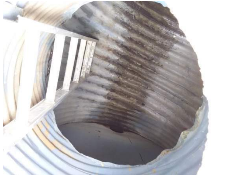
BMP #26- inside view
