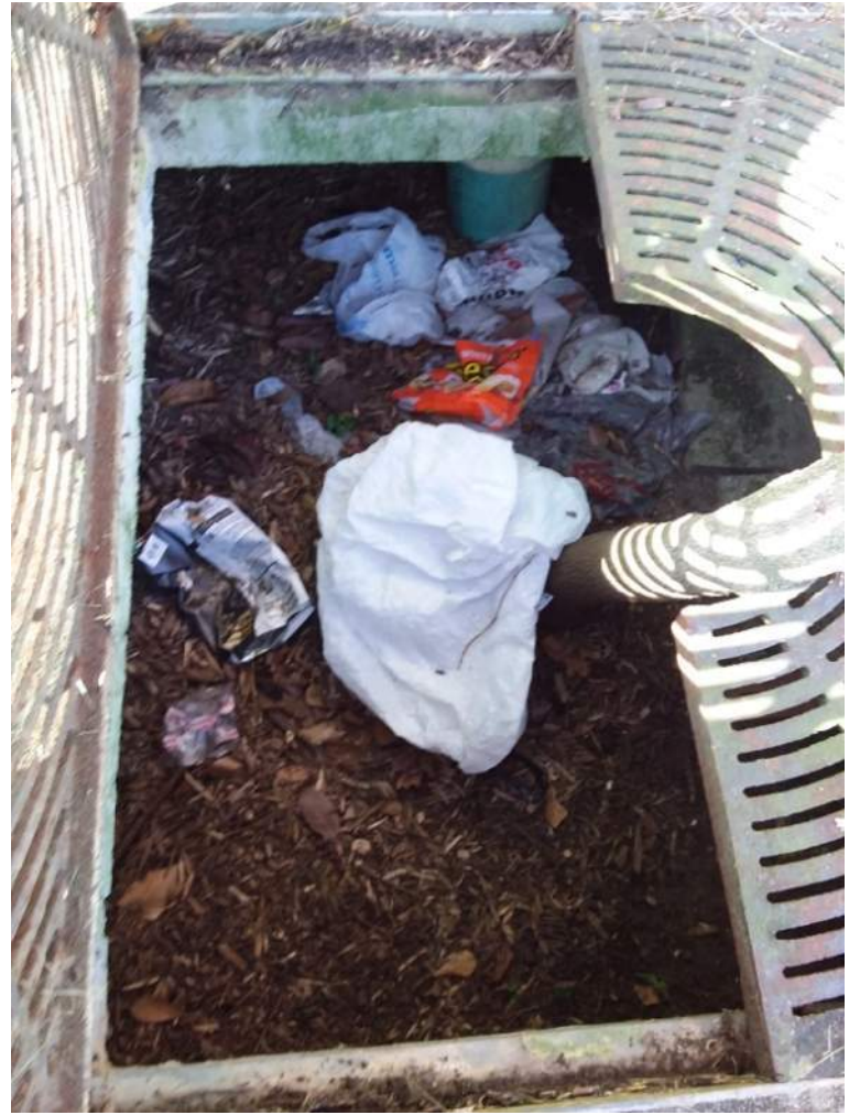
BMP #1- inside filterra
