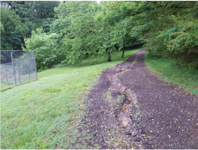
BMP #30- access road eroding and washing out
