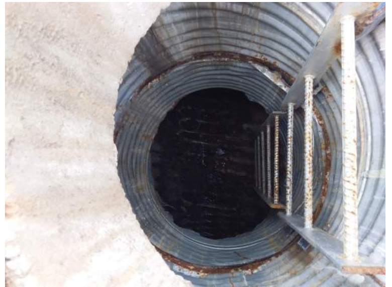
BMP #40- inside view
