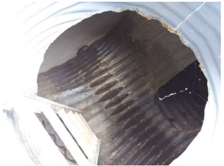
BMP #26- inside view
