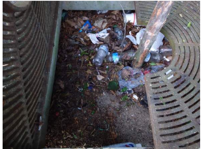
BMP #11- left side of filterra
