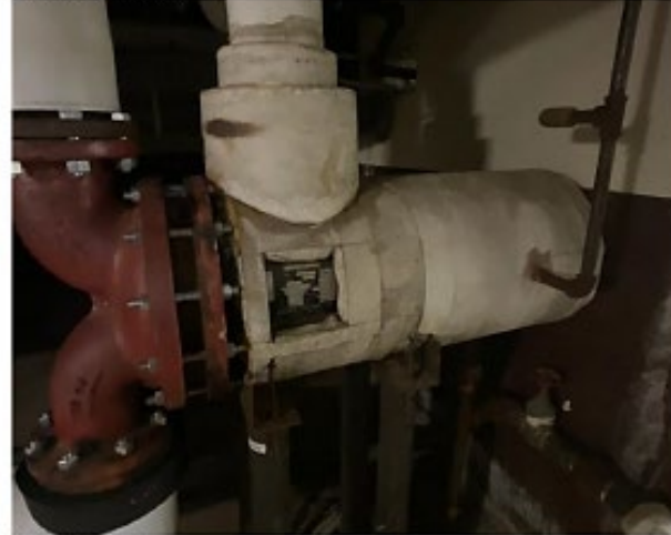
D3040 - Heat Exchanger February 28, 2023
