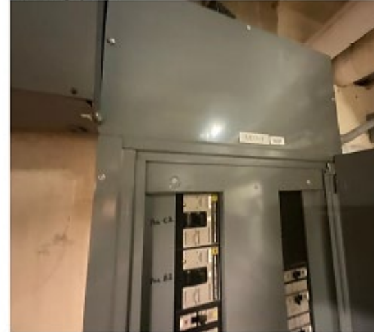
D5012 - Main Electrical Service - 1200A 208/120V February 28, 2023
