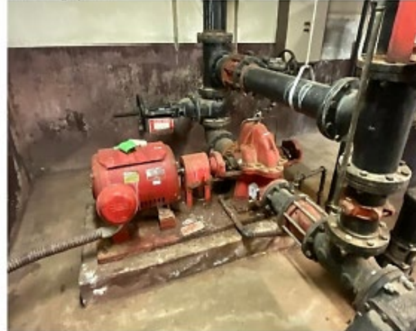
D4012 - Fire Pump - Electric - 50 HP February 28, 2023
