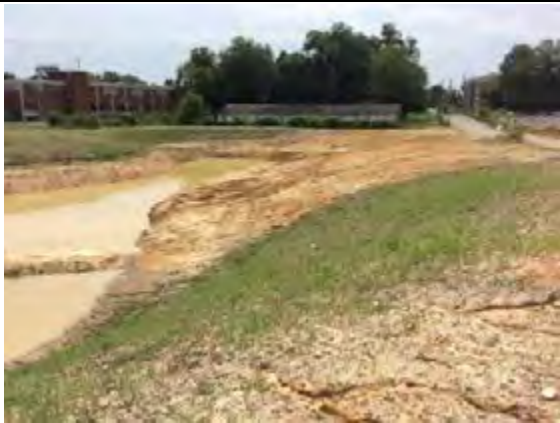
Stabilization needed on slopes
