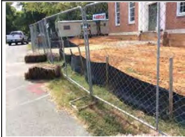
Repair holes in silt fence
