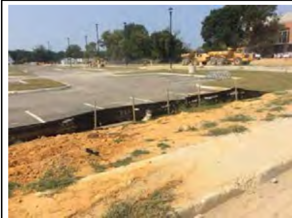
Silt fence repairs needed
