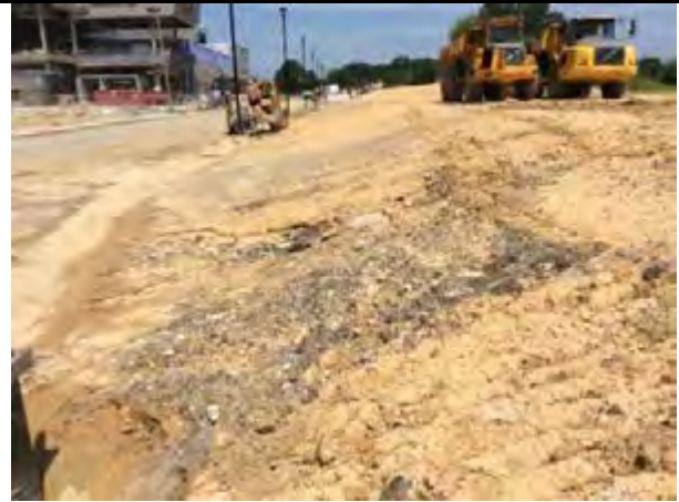
Stabilization needed, repair rills
