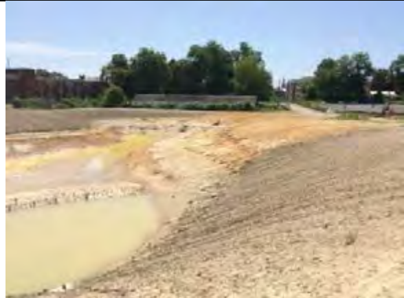
Stabilization needed on remaining slopes
