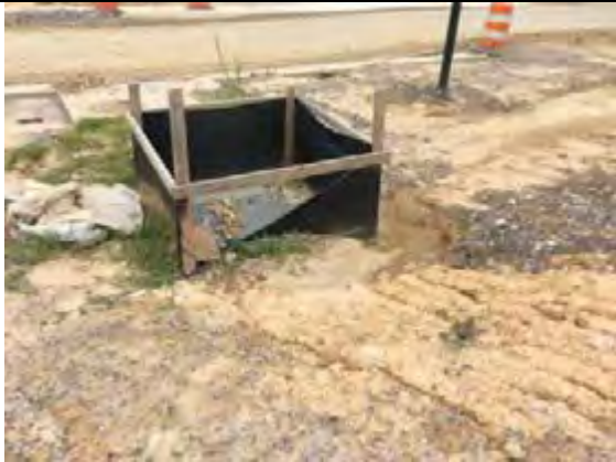
Inlet protection needs improvements
