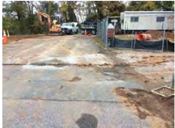
Sediment tracking in roadway
