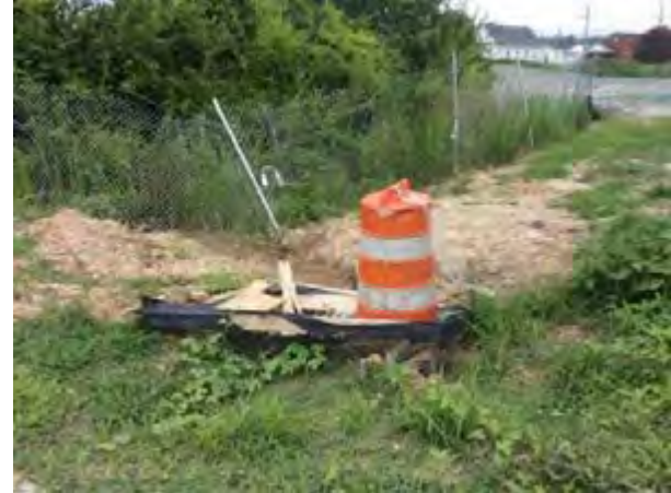
Inlet protection needs improvements
