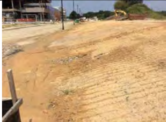
Stabilization needed on slopes
