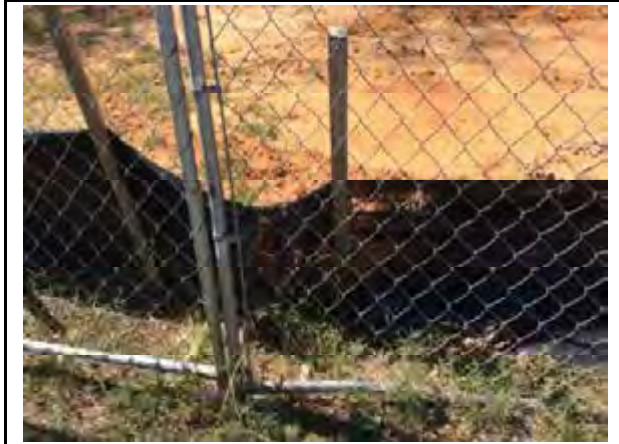
Repair holes in silt fence
