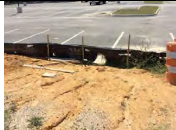
Silt fence repairs needed
