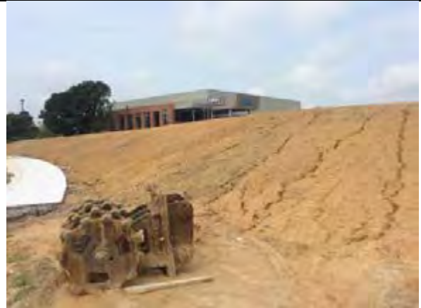
Stabilization and rill repair needed on slopes
