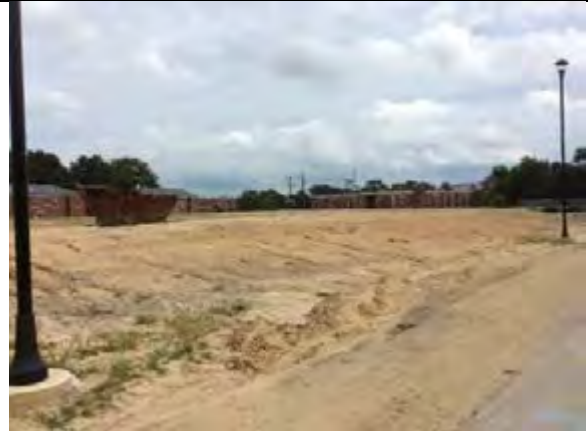
Stabilization and rill repair needed on slopes
