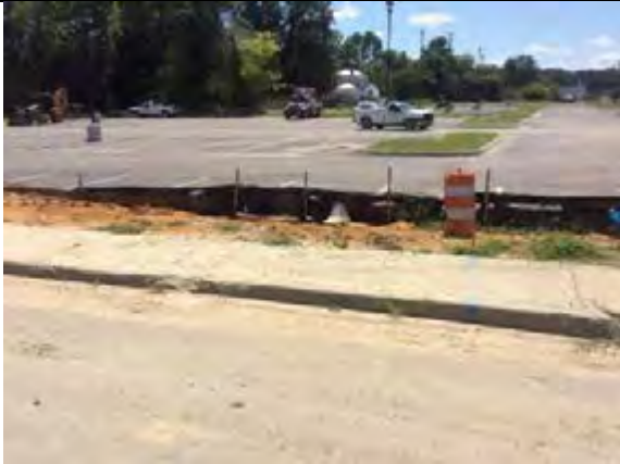
Silt fence repairs needed
