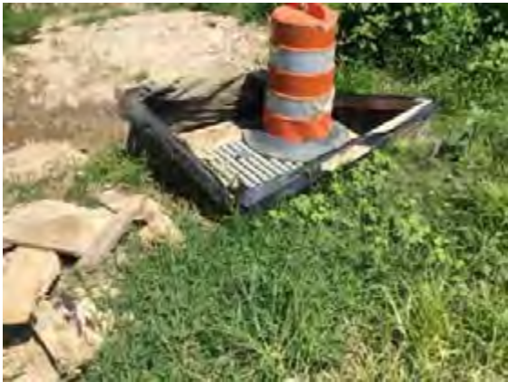
Inlet protection needs improvements
