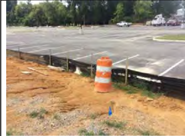
Silt fence repairs needed
