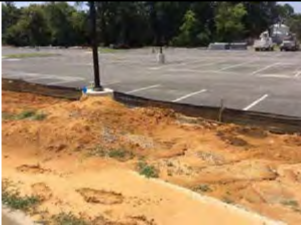
Stabilization needed and silt fence repair
