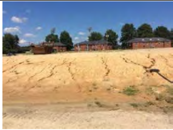
Stabilization and rill repair needed on slopes
