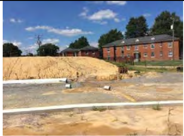
Stabilization needed and rill repair
