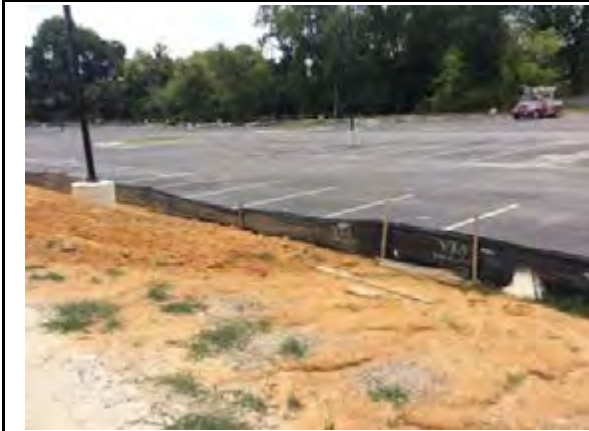
Silt fence repairs needed
