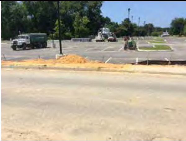
Soil needs to be placed behind silt fence
