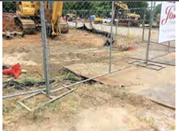
Silt fence maintenace needed
