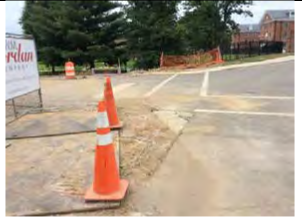
Sediment clean up needed in roadway
