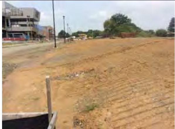
Stabilization needed and rill repair
