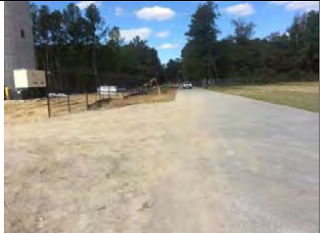
Sediment tracking in roadway
