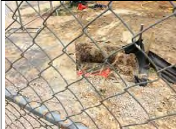
Inlet protection needs improvement
