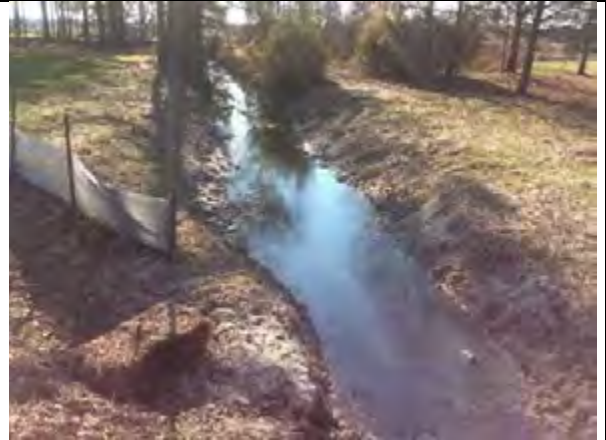
Additional stabilization needed
