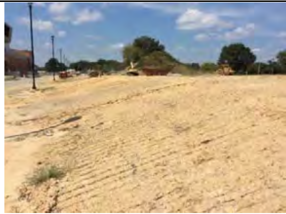
Stabilization and rill repair needed on slopes
