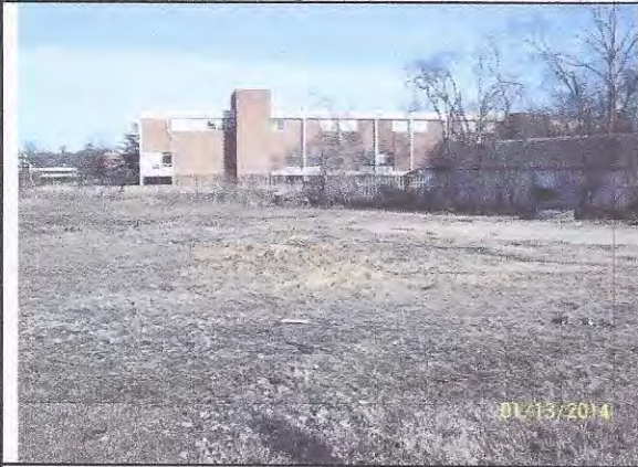
Fig. 3 – Install silt fence along the north side of the Church Property (view-east).
