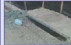
Failed Inlet Protection
